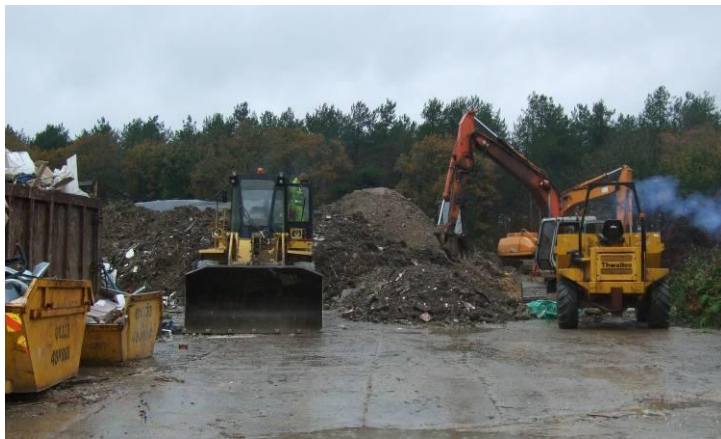
Figure A9.Site27.1: Incoming waste soil with some other wastes mixed in.
