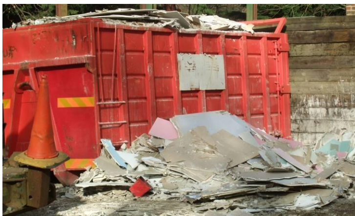
Figure A9.Site25.4: Plasterboard being stored in the open after being hand picked from mixed skips.
