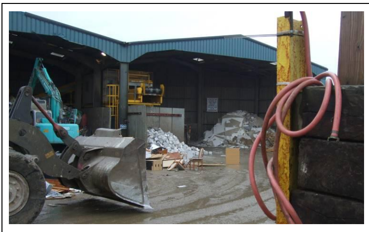
Figure A8.Site23.1: The picking station, and some stockpiles, are under cover, but in open-fronted sheds.
