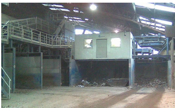
Figure A8.Site26.3: The indoor processing line for soil and aggregate. To the left are bays for the larger fractions. The picking line is in the centre.
