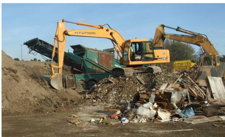
Figure A9.Site13.3: Soil / hardcore processing. To the left is a pile of screened soil, next to the excavator is a pile of incoming mixed waste containing a high proportion of inert CDEW, and to the right is general incoming mixed waste.
