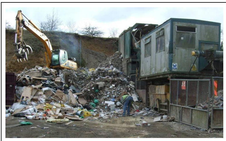
Figure A9.Site25.1: Incoming waste is tipped into one of two bays (the sleeper wall can just be seen in front of the loader, which is transferring light waste into a 'RoRo' container for onward transport). Heavy waste is fed into the trommel screen, to the right.
