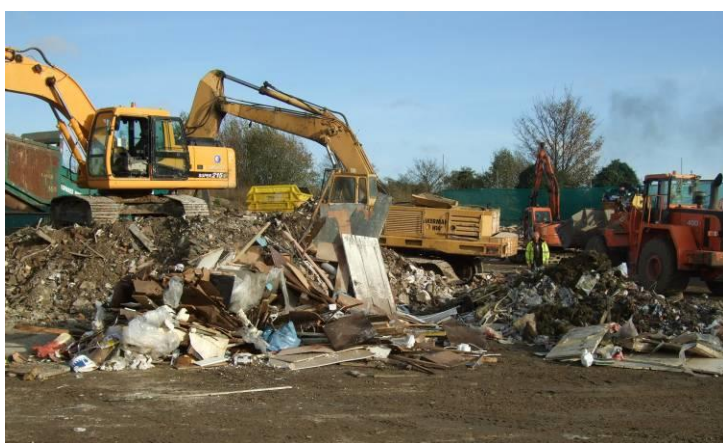
Figure A9.Site13.2: Incoming waste being hand sorted. There are three distinct loads: the pile at the back is mostly soil and hardcore, the pile in front of that is mostly wood, and the pile to the right contains a lot of green waste.
