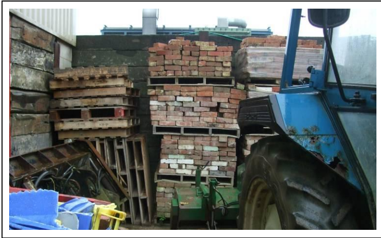
Figure A9.Site24.4: Good quality bricks and pallets extracted from CDEW, which will be sold to local companies for re-use.
