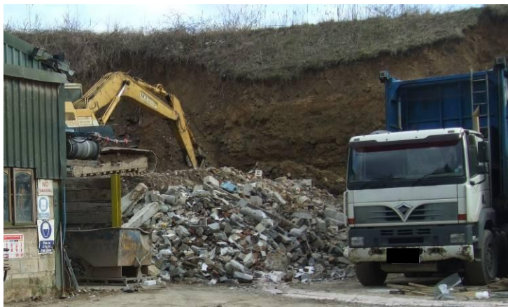
Figure A9.Site25.3: Concrete awaiting crushing. Wherever possible they crush direct into a lorry or 'RoRo' container to minimise handling costs.
