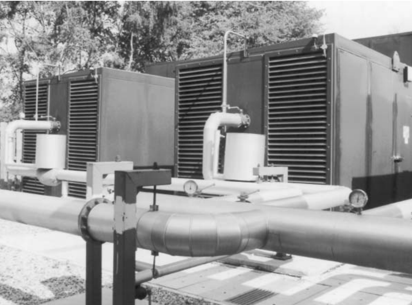
Electricity generators at Burntstump Landfill Site, Calverton. This is one of 5 landfill sites in the County where landfill gas is collected and burnt to generate electricity.
