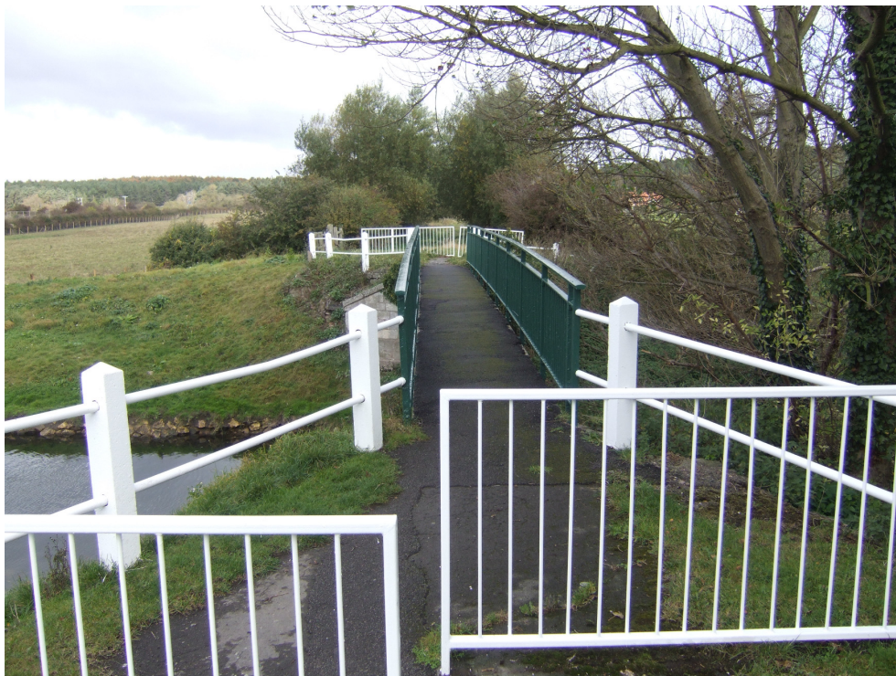
Photograph B , taken from the southern end of the footbridge over the River Idle looking north. Date of photograph 2009.
