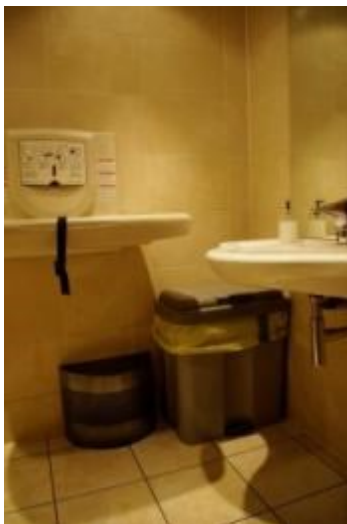
Baby changing facilities within the Accessible Toilet
