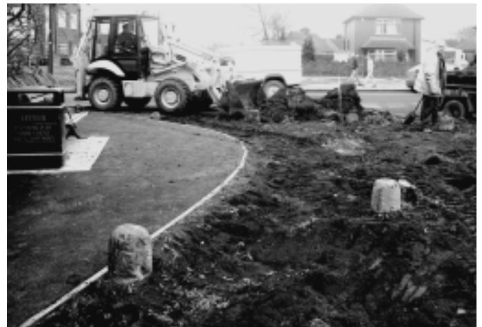
The Butterstumps undergoing renovation under the watchful eyes of Gary James and John Stevens of Mansfield District Council.
